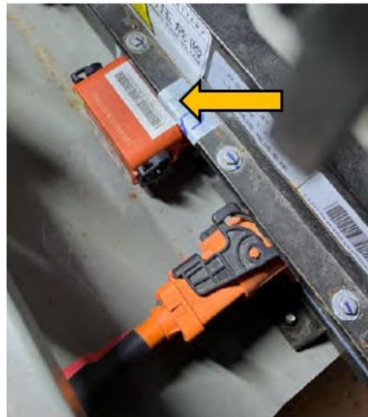
Image: MSD located on the front side of the high-voltage battery, next to HV cables.
