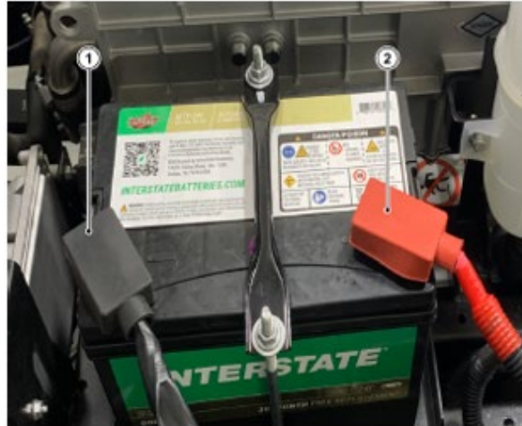
Image: 12-Volt Battery Terminals
